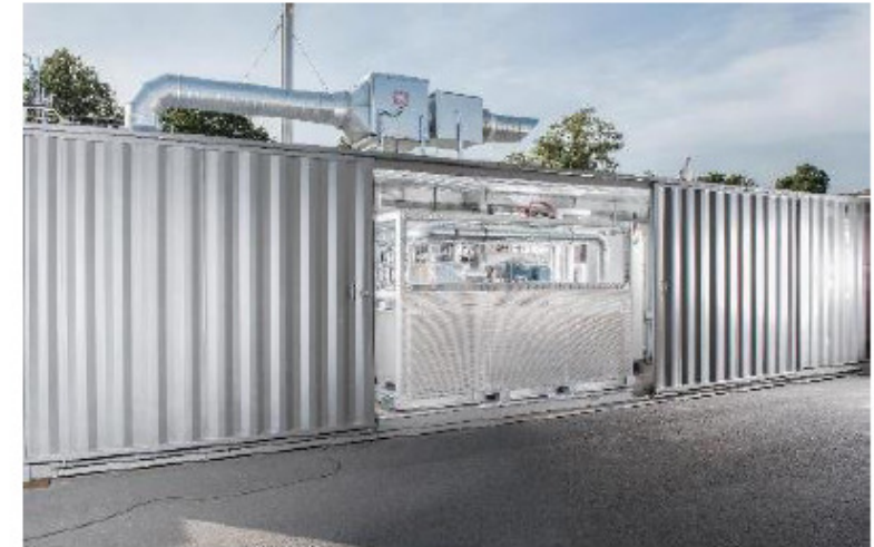
150 kW SOEC unit in Salzgitter, Germany
